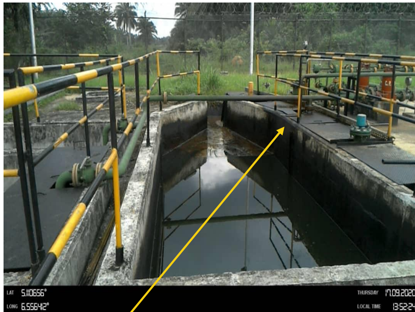
Close-up: Overflow Saver pit on Ubie Flow Station at Idu-Ekpeye . Picture was taken during Joint Investigation on 17th September 2020.
