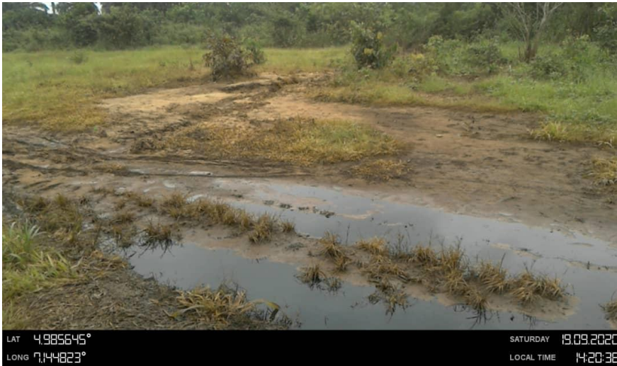
Overview: Part of spill impact on 8" Nkali - Imo River2 Delivery line at Muanyimochi-Odagwa. Picture was taken during Joint Investigation on 19th September 2020.
