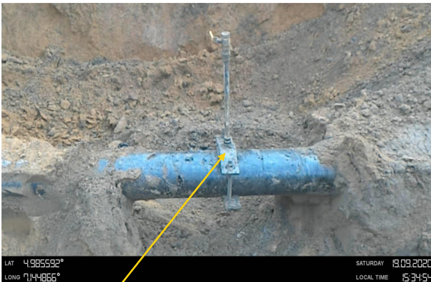
Close-up: Crude oil theft point installed at 9 o'clock position on 8" Nkali - Imo River2 Delivery line at Muanyimochi-Odagwa. Picture was taken during Joint Investigation on 19th September 2020.
