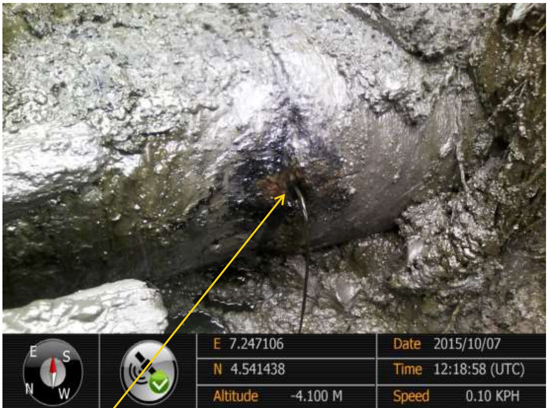
Close-up: Spill due to corrosion on 24" Bomu-Bonny Pipeline at Owokiri. Picture was taken during Joint Investigation of 7 th October 2015.
