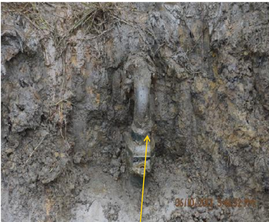
Close up: Spill point 2 - due to illegal fitting 20" Otumara Escravos Pipeline at Ajudaibo. Picture was taken during Joint Investigation of 6th October 2013.
