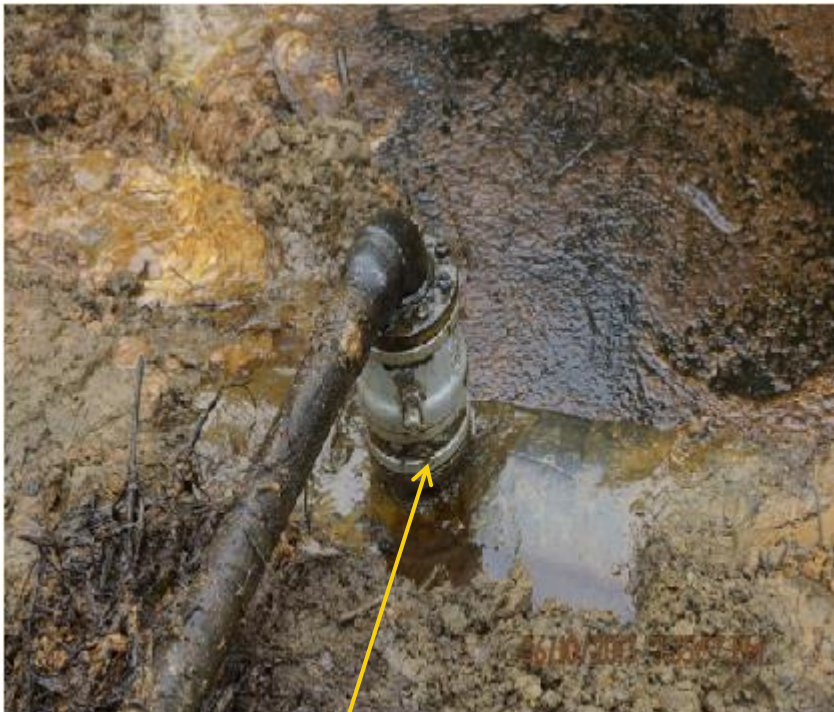
Close up: Spill point 1 due to illegal fitting 20" Otumara Escravos Pipeline at Ajudaibo. Picture was taken during Joint Investigation of 6th October 2013..
