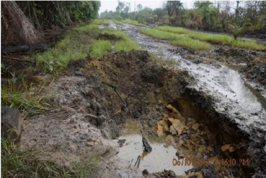
Overview: Part of spill point 1 impact on 20" Otumara Escravos Pipeline at Ajudaibo. Picture was taken during Joint Investigation of 6th October 2013.
