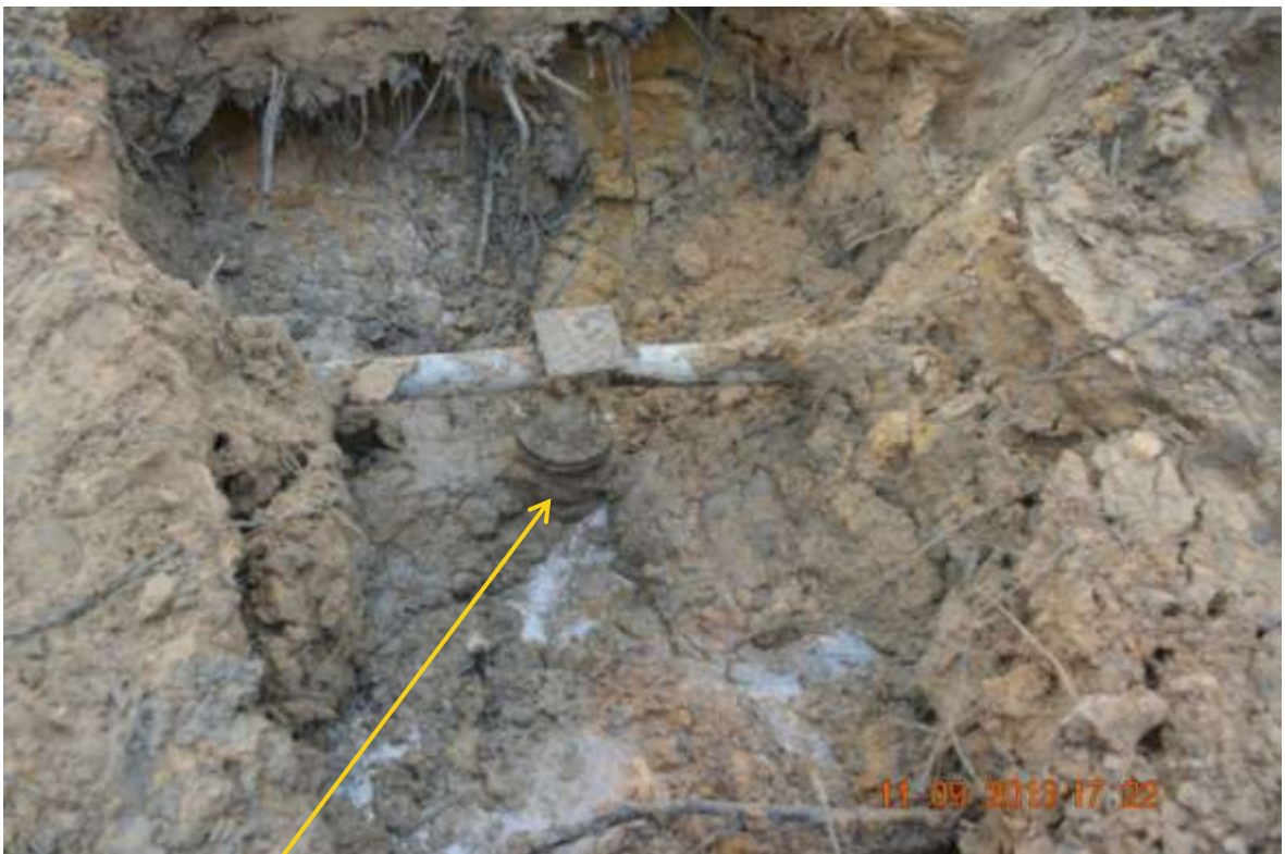
Close up: Illegal fitting 20" Otumara-Escravos pipeline at Ugborodo/Ugboegungun. Picture was taken during Joint Investigation of 11 th September 2013.
