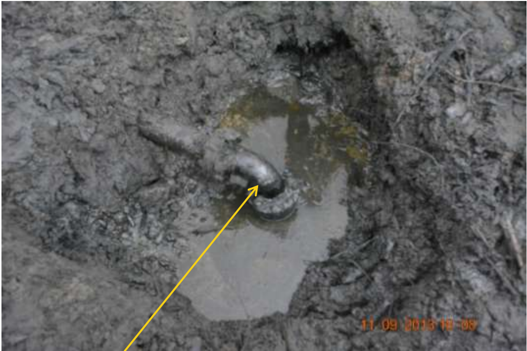
Close up: Illegal fitting on 20" Otumara-Escravos pipeline at Ugborodo/Ugboegungun. Picture was taken during Joint Investigation of 11 th September 2013.
