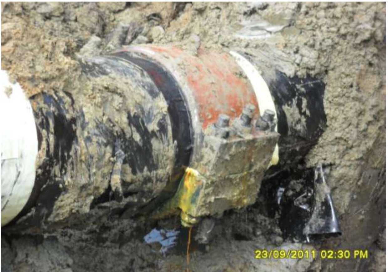
Close-up: Spill due to failed dam on 20" Kolocreek–Rumuekpe Pipeline at Ogbogolo. Picture was taken during JIV of 23 rd September, 2011
