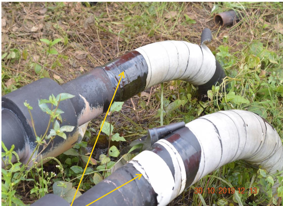
Close-up: Hack Saw Cuts on 4" Agbada2 Well 58 Flowline at Omueke. Picture was taken during Joint Investigation of 30 th October 2019.
