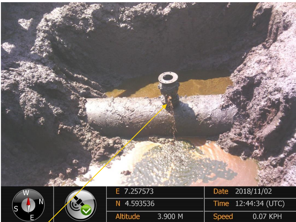
Close up: Illegal fitting on 24" Bomu-Bonny Pipeline at Patrick Waterside. Picture was taken during Joint Investigation of 2 nd November 2018.
