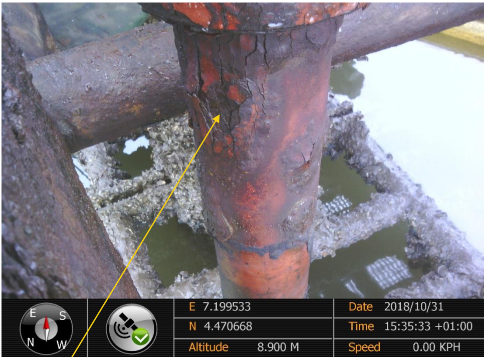
Close up: Impacted Section on 4" Bonny Well 18S Flowline Riser at Oloma. Picture was taken during Joint Investigation of 31 st October 2018.
