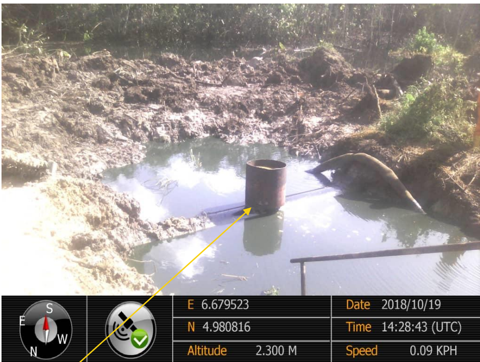
Close up: Illegal fitting on 20" Kolocreek-Rumuekpe Pipeline at Imogu-Rumuekpe. Picture was taken during Joint Investigation of 19 th October 2018.
