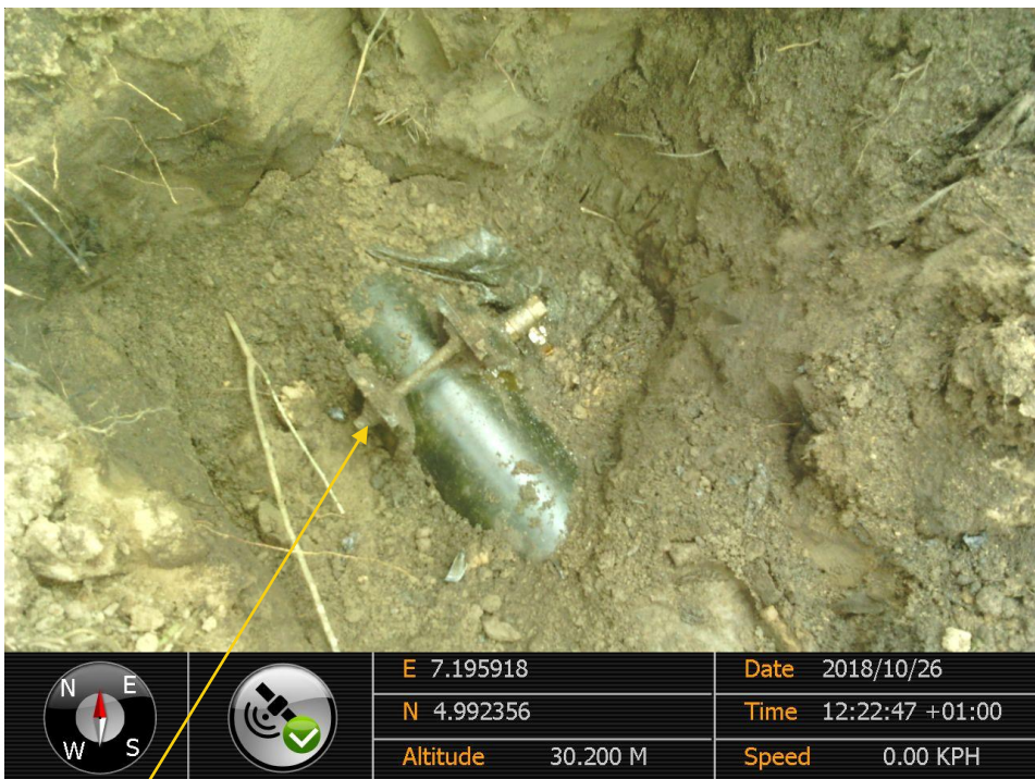
Close up: Illegal fitting on Imo River1–Well 37 Flowline at Igiriukwu-Owaza. Picture was taken during Joint Investigation of 26 th October 2018.
