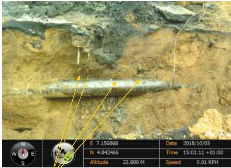
Close up: Illegal fittings on 12" Imo River – Ogale Pipeline at Okpa-Umuakpahu. Picture was taken Joint Investigation of 3rd October 2018.
