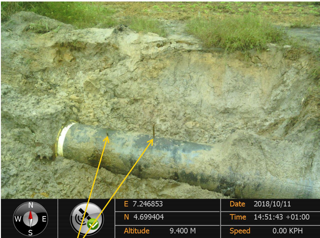
Close up: Drilled Holes on 28" Nkpoku-Bomu Pipeline at Gio. Picture was taken during Joint Investigation of 11th October 2018.
