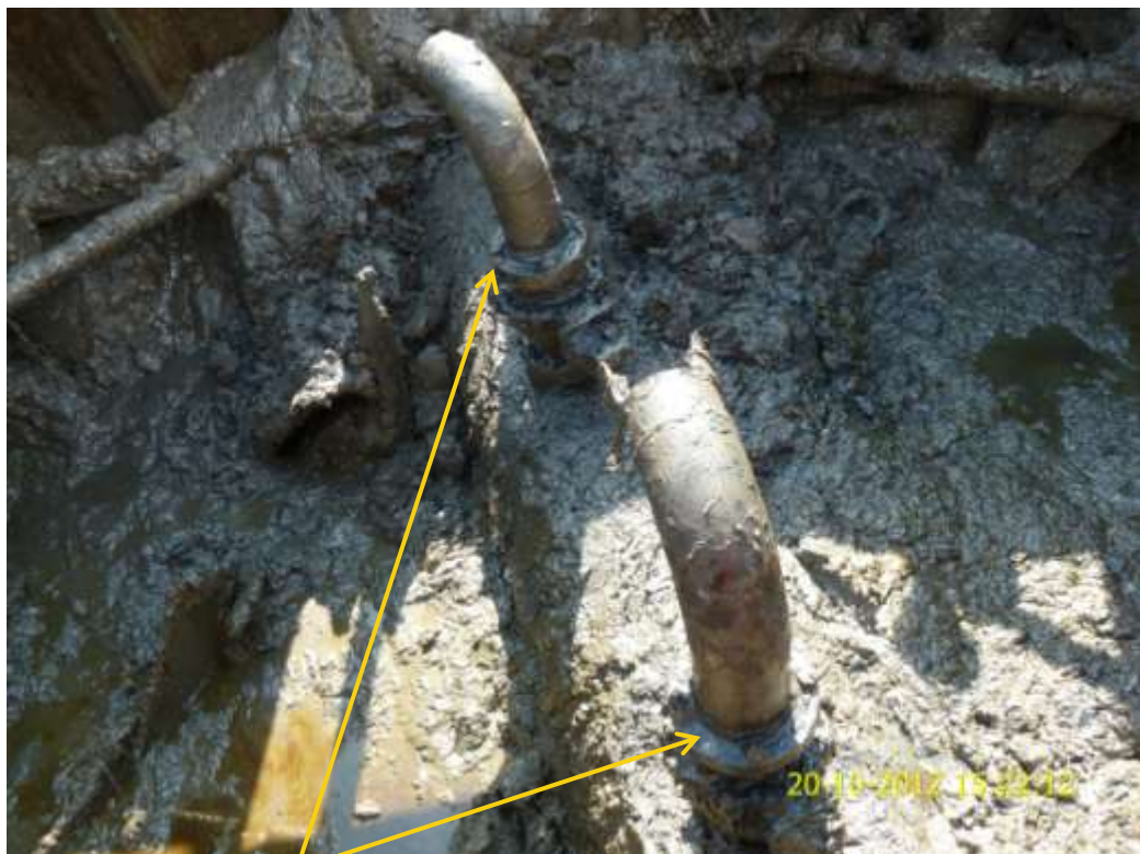
Close up: Illegal fittings on 28" Bomu-Bonny Tran Niger pipeline at Okolo. Picture was taken during Joint Investigation of 20 th October 2012.
