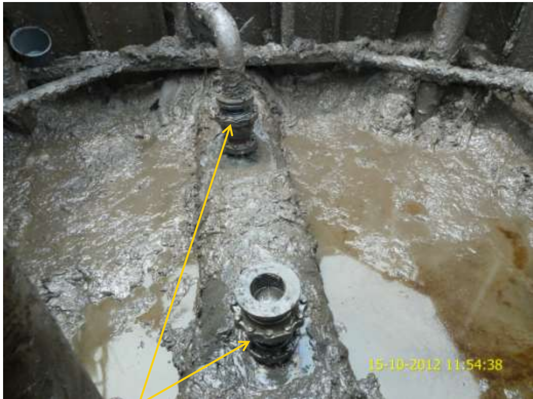
Close up: Illegal fittings on 28" Bomu-Bonny Tran Niger pipeline at Okolo. Picture was taken during Joint Investigation of 15 th October 2012.
