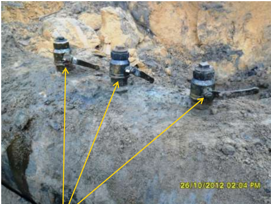
Close up: Illegal fittings on 28" Nkpoku-Bomu pipeline at Aleto. Picture was taken during Joint Investigation of 26 th October 2012.
