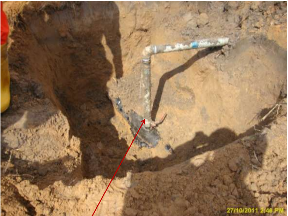
Close-up: Illegal fitting on 6" Obigbo North – Ogale pipeline at KomKom. Picture was taken during Joint Investigation of 27th October, 2011.
