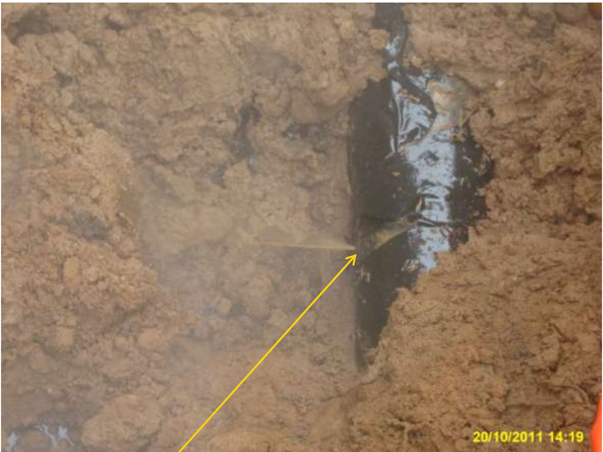
Close-up: Hack saw cut on 6" Obigbo – North Pipeline at Ogale. Picture was taken during Joint Investigation of 20th October 2011.
