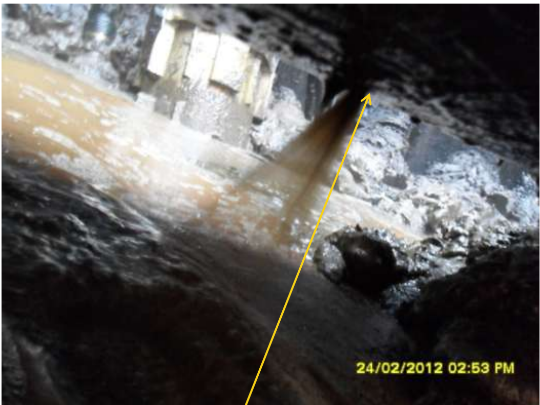
Close up: Spill point at 6 'o clock position on 28" Awoba-Cawthorne Channel pipeline right of way at Brigede. Picture was taken during Joint Investigation of 24 th February 2012.
