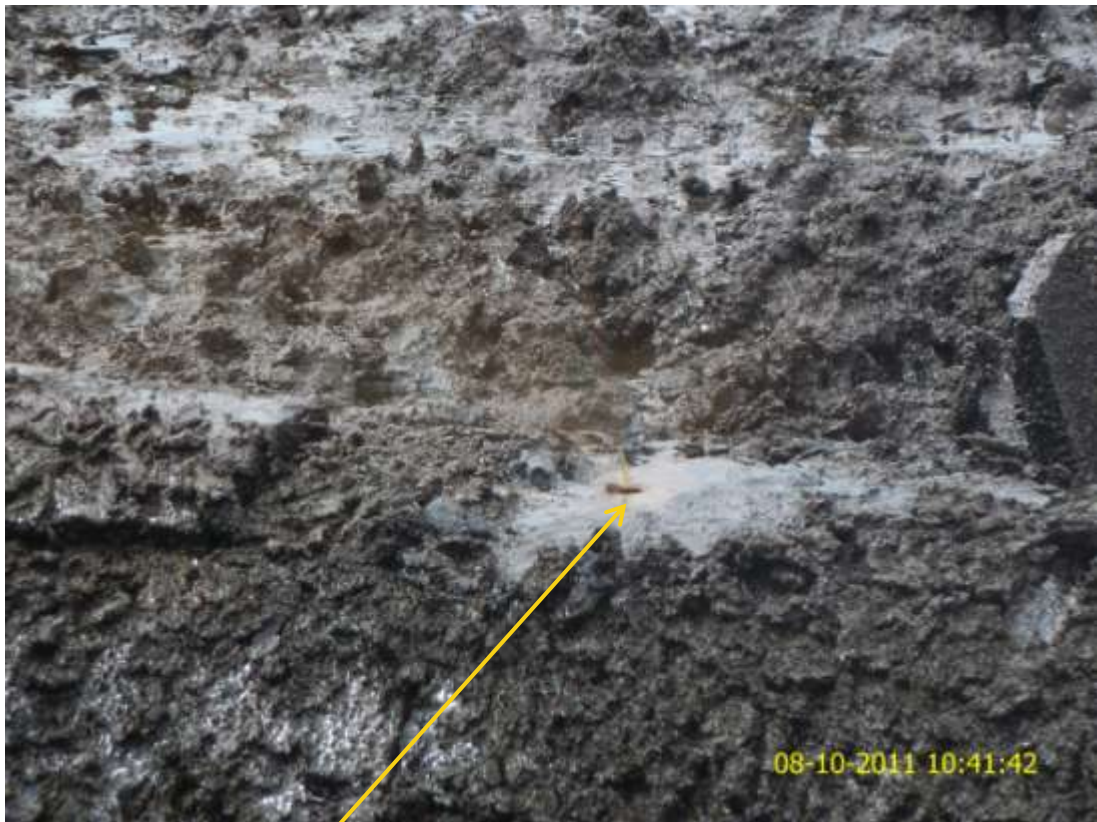
Close-up: Drilled hole on 24" Alakiri-Bonny pipeline right of way at Ilomaturu. Picture taken during Joint Investigation of 8 th October, 2011.
