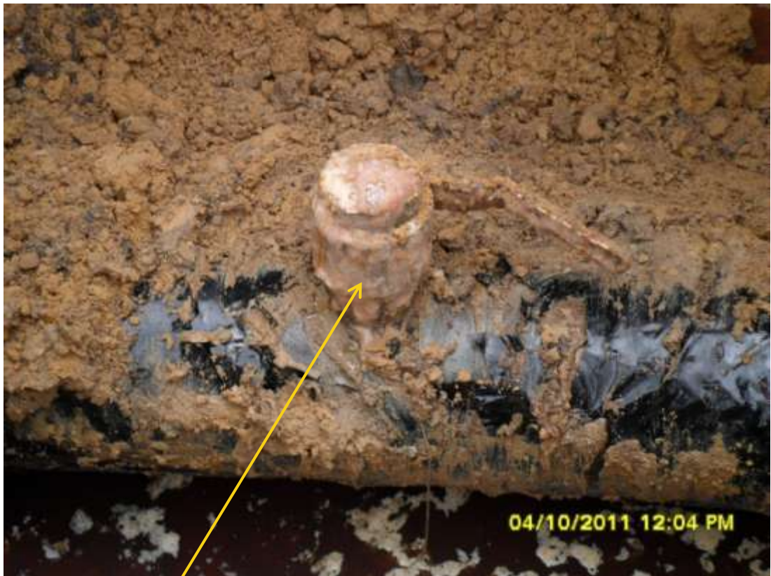
Close-up: Illegal fitting on 6" Obigbo North pipeline at KomKom. Picture taken during Joint Investigation of 4 th October, 2011
