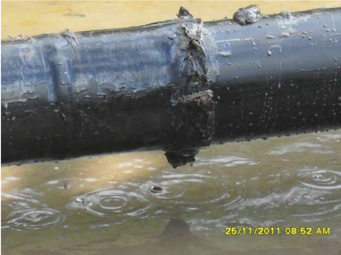
Close-up: Spill due to pinhole and slight tear close to previous weld on Kanbo Well 5L flowline at Egbemo Angalabiri. Picture taken during Joint Investigation of 25 th November 2011.
