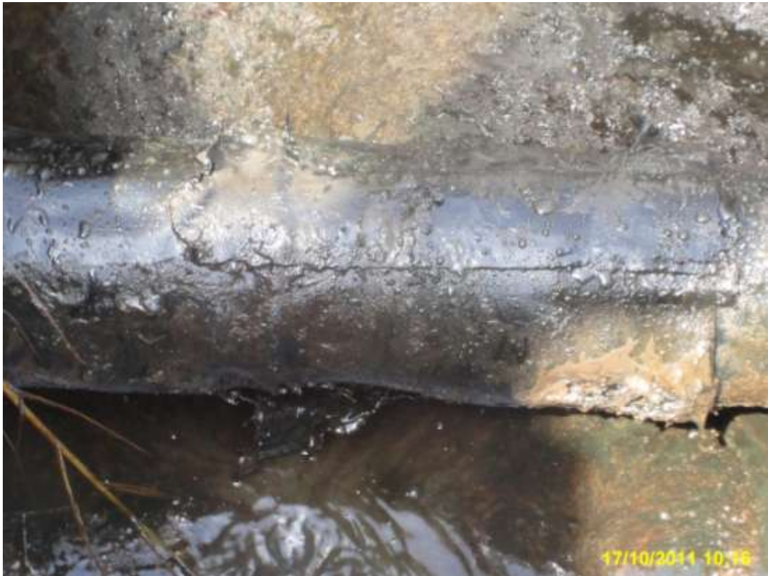
Close-up: Spill due to corrosion on Cawthorne Channel2 Well51T flowline at Mbiama. Picture taken during Joint Investigation of 17 th October, 2011.
