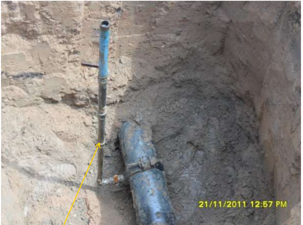
Close-up: Illegal fitting on 8" Nkali-Imo River2 pipeline at Odagwa. Picture was taken during Joint Investigation of 21 st November, 2011.
