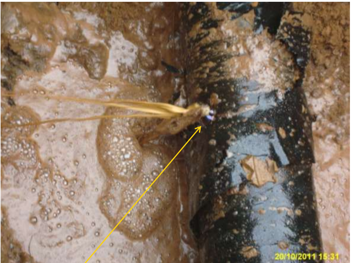
Close-up: Hacksaw cut on 6" Obigbo – North Pipeline at Ogale. Picture was taken during Joint Investigation of 20th October, 2011.
