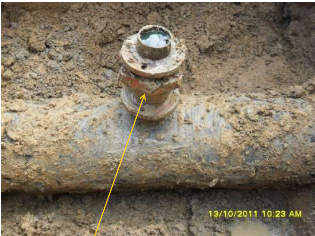
Close-up: Illegal fitting discovered after excavation on 12" Egbema-Oguta pipeline at Eziosu. Picture taken during Joint Investigation of 13 th October, 2011.
