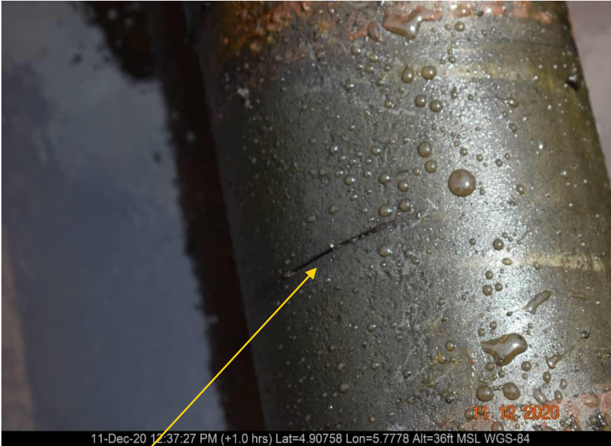
Close-up: Hack Saw Cut on 6'' Seibuo Well 3 & 4 Bulkline at Agbidiana. Picture was taken during Joint Investigation on 11 th December 2020.
