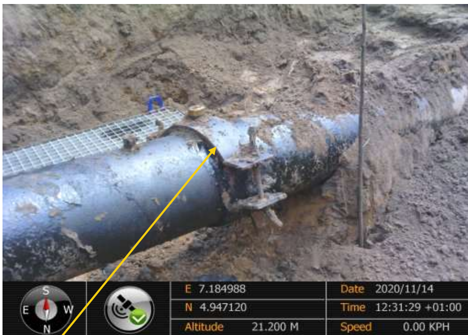
Close-up: Locally fitted clamp with 1.5inch valve installed at 12 o'clock position on 12inch Imoriver 1 - Ogale Pipeline at Umulolo. Picture was taken during Joint Investigation on 14th November 2020.
