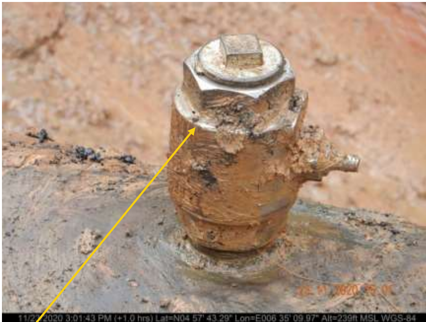
Close-up: 2inch valve installed at 12 o'clock position on 20inch Kolocreek – Rumuekpe Trunkline at Owerewere. Picture was taken during Joint Investigation on 23rd November 2020.
