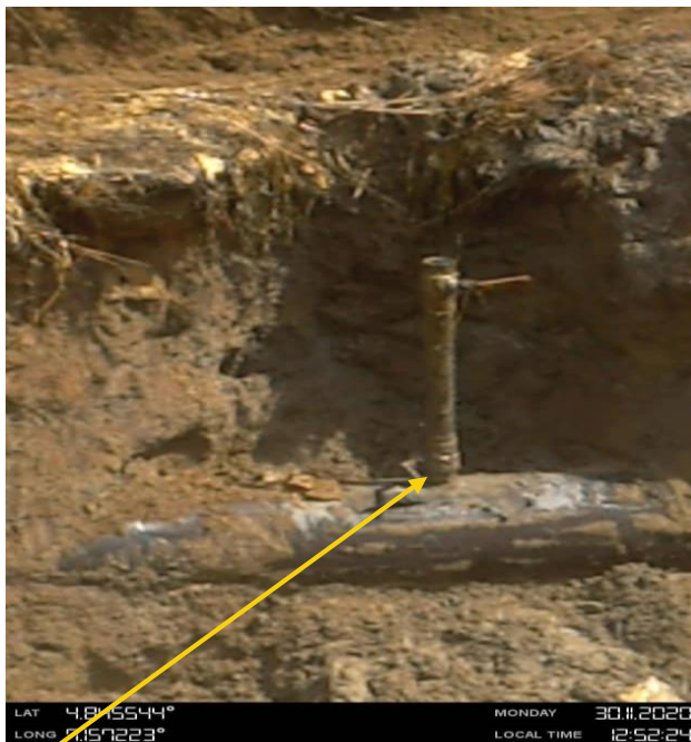
Close-up: 1.5inch pipe fitted with 2nos of 1.5inch valves installed at 12 o'clock position on 12'' Imoriver 1 - Ogale Pipeline at Komkom. Picture was taken during Joint Investigation on 30th November 2020.
