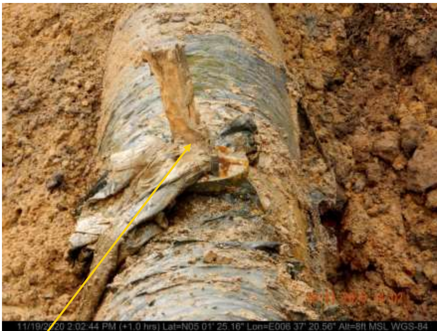
Close-up: Plugged 2inch Ball valve installed at 12 o'clock position on 14inch Okordia Rumuekpe Trunkline at Edeoha. Picture was taken during Joint Investigation on 19th November 2020.
