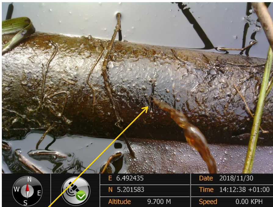
Close-up: Hacksaw Cut on 4" Adibawa Well 12T Flowline at Edagberi. Picture was taken during Joint Investigation of 30 th November 2018
