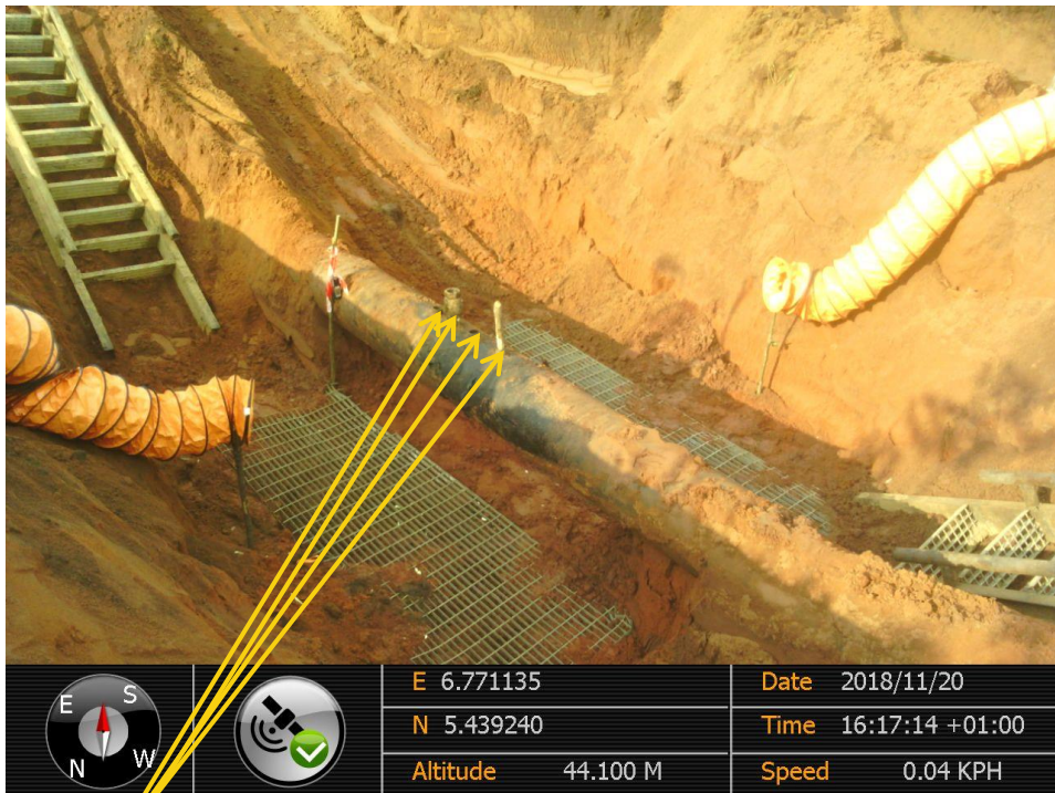
Close-up: Illegal fittings on 16" Egbema - Assa Pipeline at Umudike. Picture was taken during Joint Investigation of 20 th November 2018.
