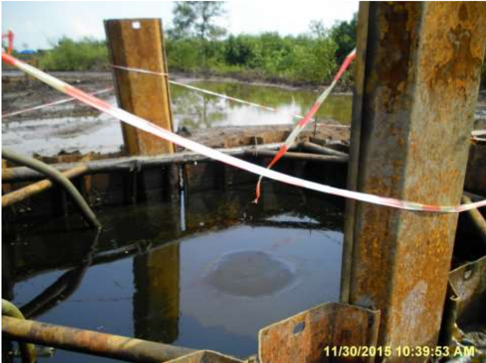
Overview: Part of spill impact on 28" Bomu-Bonny Pipeline at Otokolomabie/Oloma. Picture was taken during Joint Investigation of 30 th November 2015.
