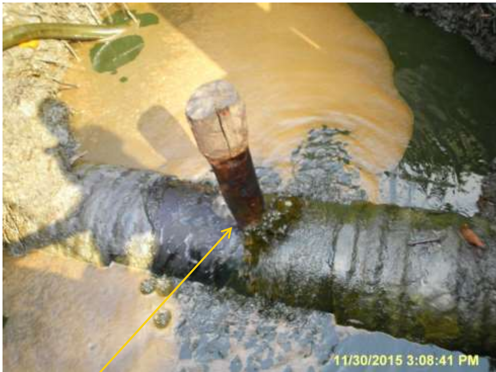
Close-up: Position of illegal fitting after removal on 28" Bomu-Bonny Pipeline at Otokolomabie/Oloma. Picture was taken during Joint Investigation of 30 th November 2015.
