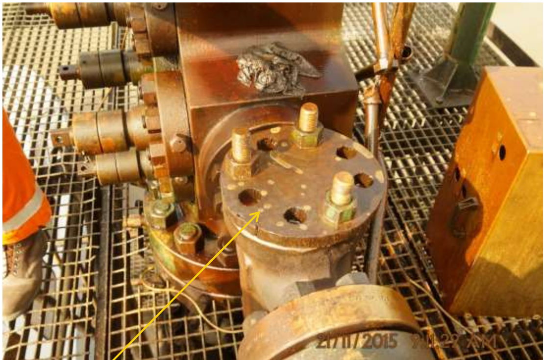
Close-up: Original position of Cameron Control Unit on Tunu Kanbo Well4L Wellhead at Agbidiana . Picture was taken during Joint Investigation of 21 st November 2015.
