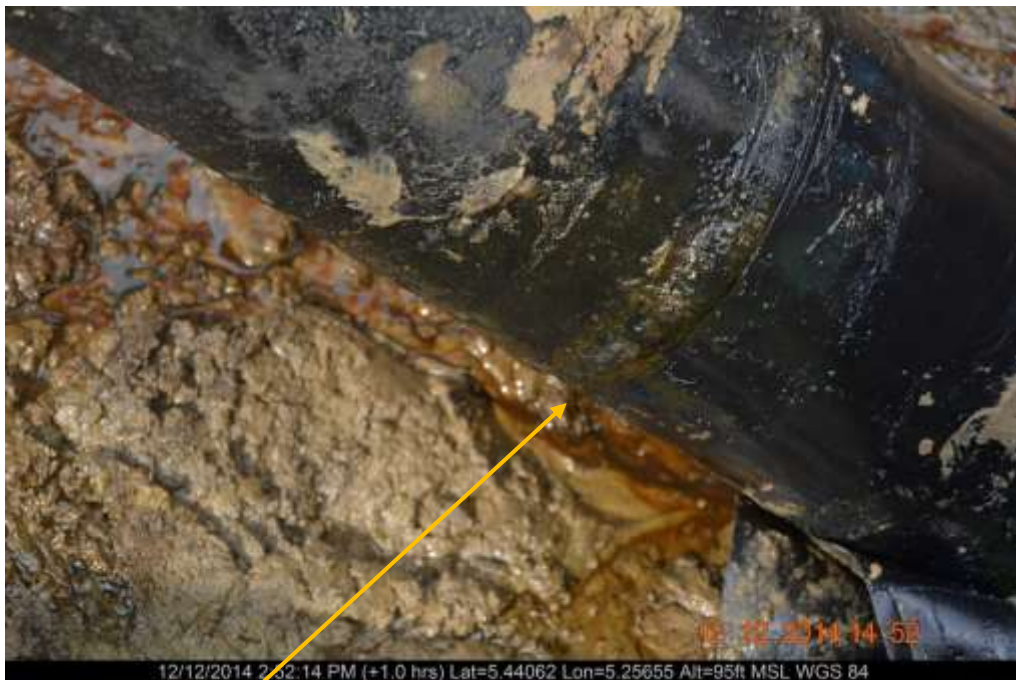
Close-up: Spill point on 6" Yokri Manifold7 Test Flowline at Yokri. Picture was taken during Joint Investigation of 12 th of December 2014.
