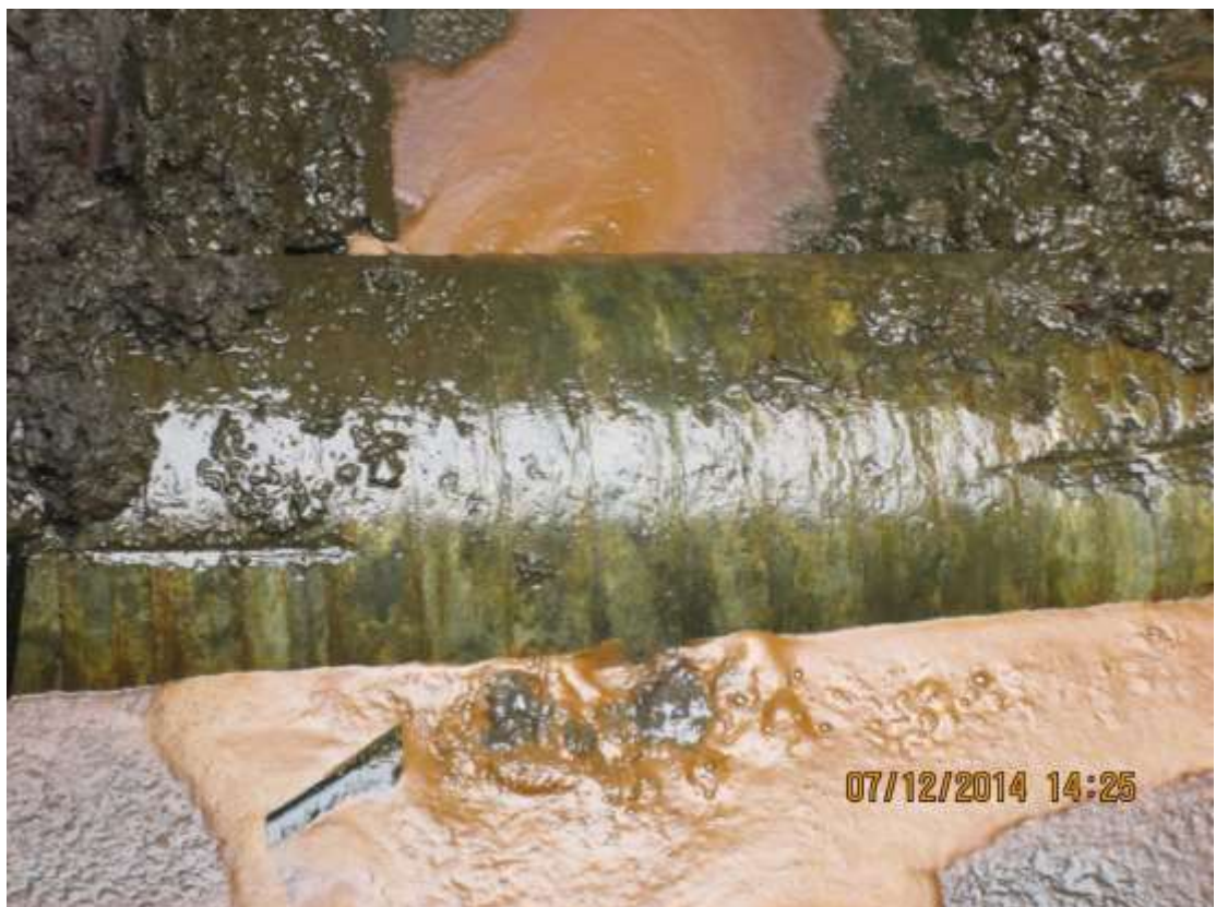
Close-up: Spill due to corrosion on 24" Tora - Segoo Pipeline at Segoo. Picture was taken during Repair Operation of 7 th December 2014.
