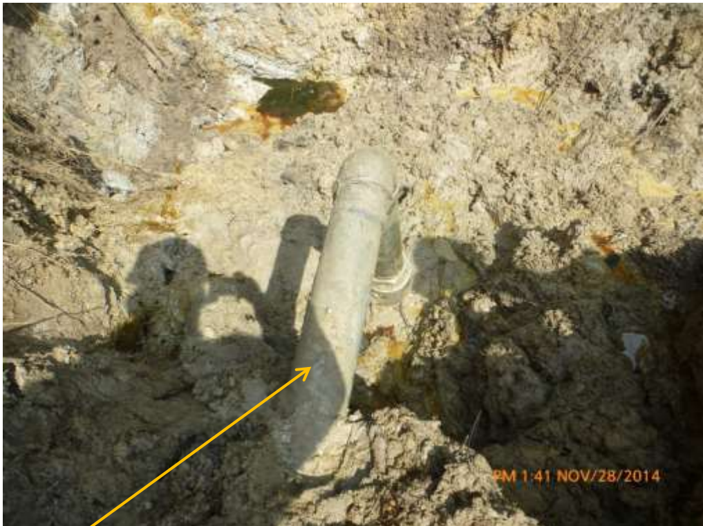
Close-up: Illegal fitting on 28" Bomu-Bonny Pipeline at Mogho. Picture was taken during Joint Investigation of 28 th November 2014.
