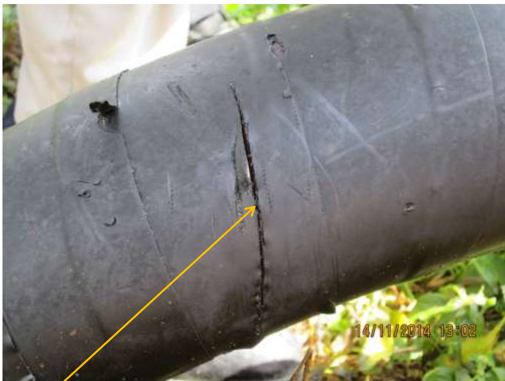
Close-up: Hacksaw cut on Ahia Well3SL Flowline at Egbeda. Picture was taken during Joint Investigation of 14 th November 2014.
