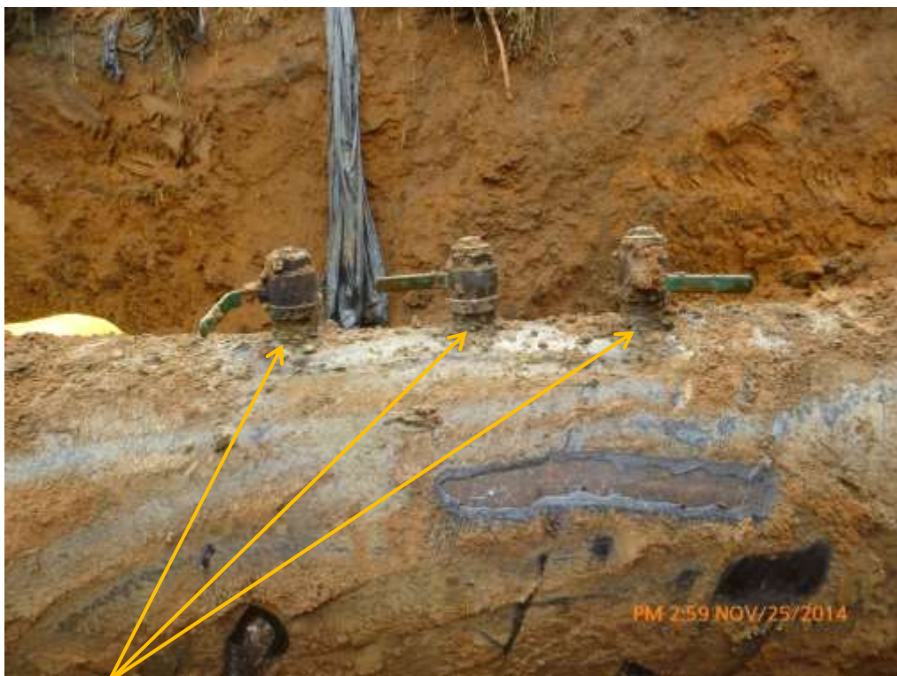
Close-up: Illegal fittings on 28" Nkpoku-Bomu Pipeline at Elenwo. Picture was taken during Joint Investigation of 25 th November 2014.
