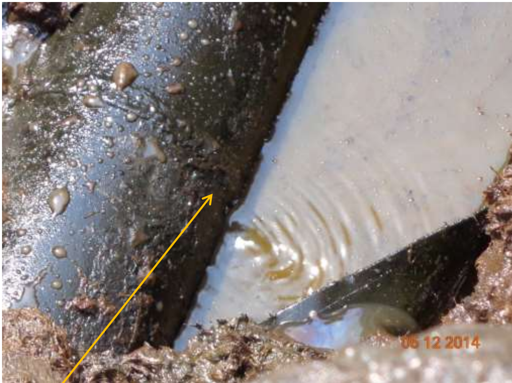
Close-up: Failed weld on Ekulama 2 Well24T Flowline at Freetown. Picture was taken during Joint Investigation of 5 th December 2014.
