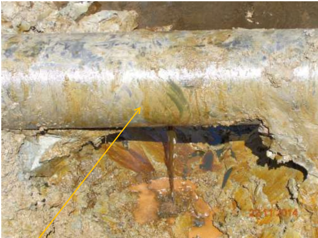
Close-up: Spill due to corrosion on 14" Okordia-Rumuekpe Pipeline at Ikarama. Picture was taken during Joint Investigation of 22 nd November 2014.
