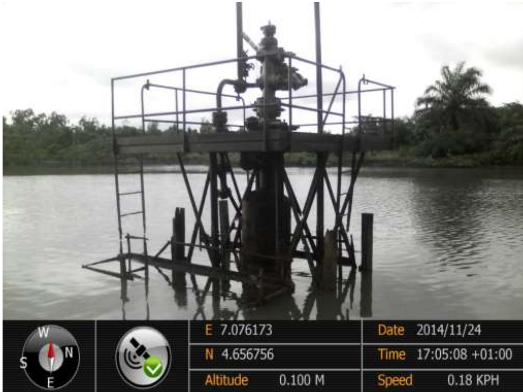
Overview: Spill point on Alakiri Well19T Wellhead Right of Way at Ofiomina-Ama. Picture was taken during Joint Investigation of 24 th November 2014.
