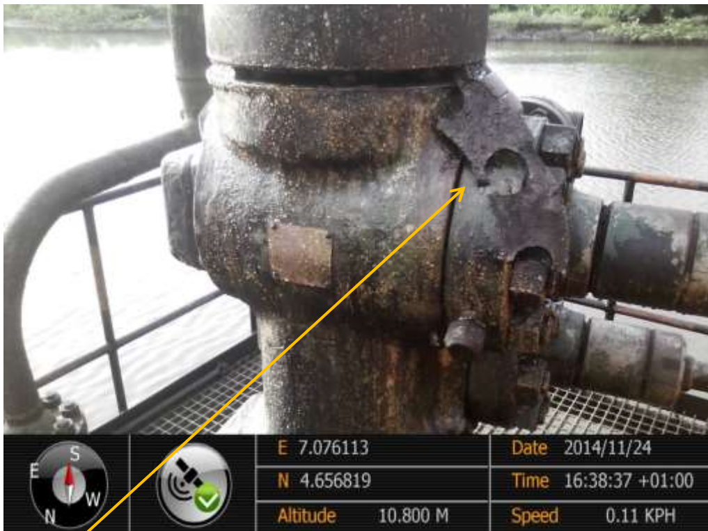
Close-up: Exposed internal thread tape on Alakiri Well19T Wellhead at Ofiomina-Ama. Picture was taken during Joint Investigation of 24 th November 2014.
