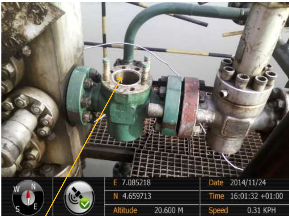
Close-up: Position of missing Surface Safety Valve actuator on Alakiri Well31L Wellhead at Ofiomina-Ama. Picture was taken during Joint Investigation of 24 th November 2014.
