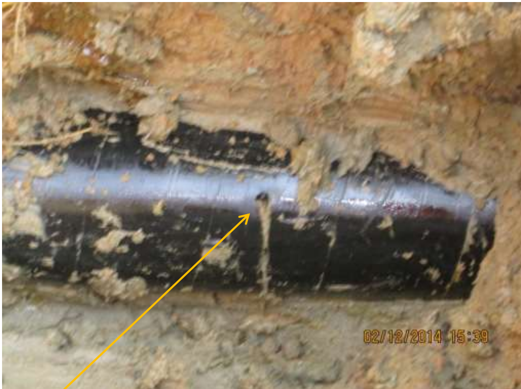
Close-up: Hacksaw cut on 4" Etelebou Well 11T Flowline at Ogboloma. Picture was taken during Joint Investigation of 2 nd December 2014.
