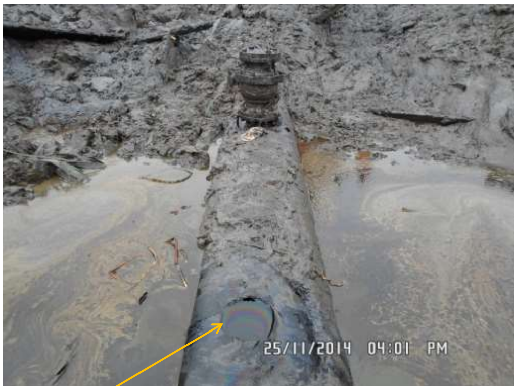
Close-up: Position of failed illegal fitting on 24" Bomu-Bonny Pipeline at Okolo Launch. Picture was taken during Joint Investigation of 25 th November 2014.
