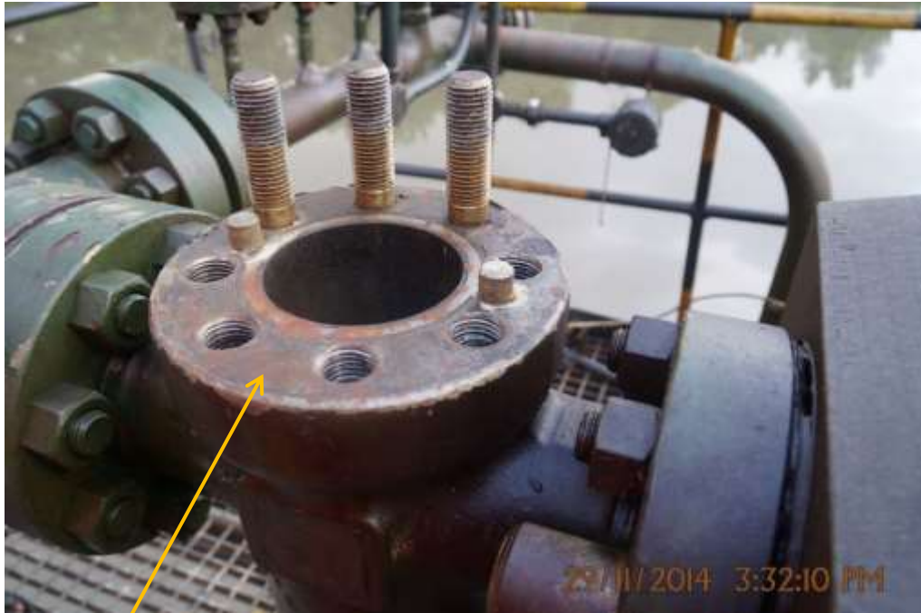
Close-up: Location of stolen Control Unit (Well-4S) on Tunu Wellhead 4LS at Bilabiri. Picture was taken during Joint Investigation of 29 th November 2014.
