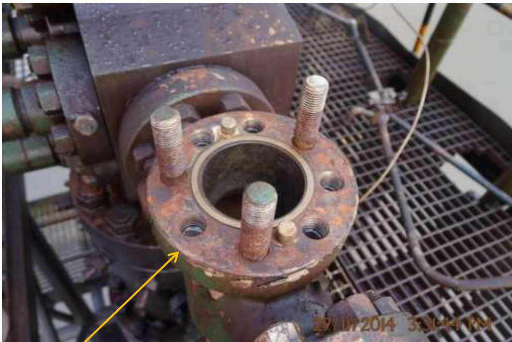
Close-up: Location of stolen Control Unit (Well-4L) on Tunu Wellhead 4LS at Bilabiri. Picture was taken during Joint Investigation of 29 th November 2014.
