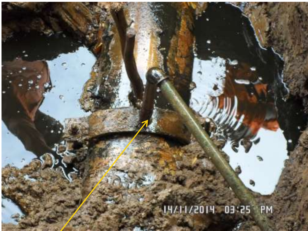
Close-up: Illegal fitting on 12" Imo River2 – Ogale Pipeline at Owaza. Picture was taken during Joint Investigation of 14 th November 2014.
