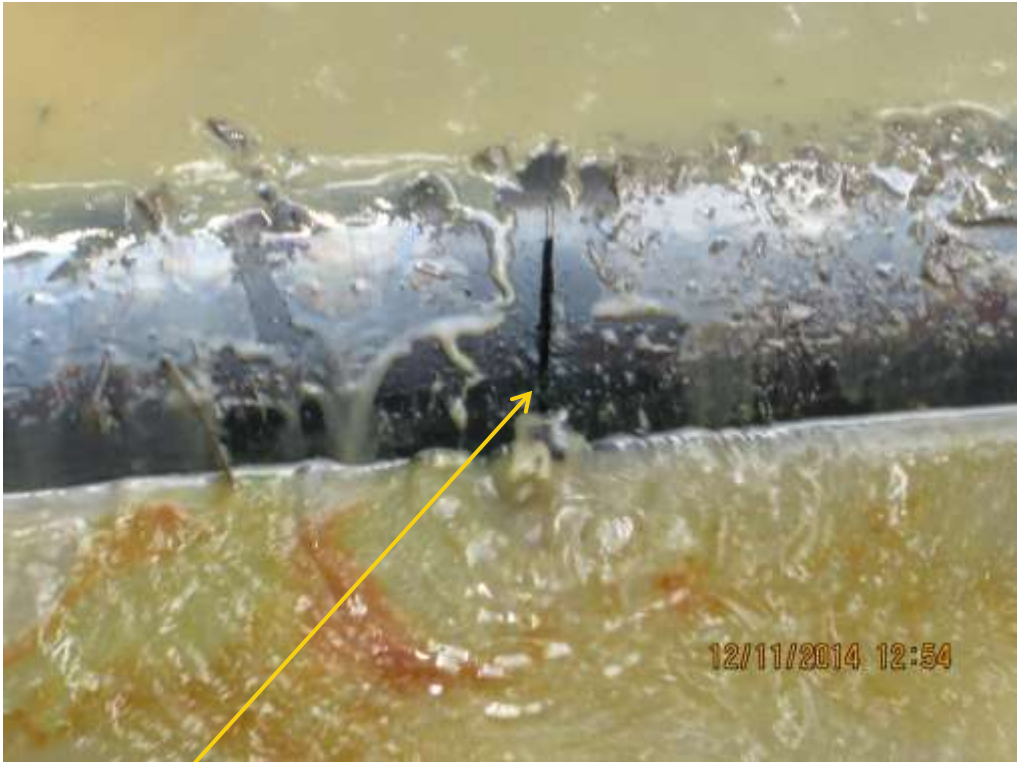
Close-up: Hacksaw cut on Kolo Creek Well3T Flowline at Otuasega. Picture was taken during Joint Investigation of 12 th November 2014.
