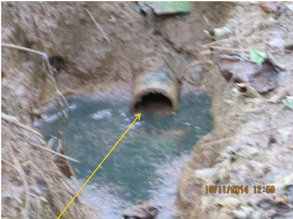
Close-up: Cut section on 4" Ahia Well3S Flowline at Egbeda. Picture was taken during Joint Investigation of 18 th November 2014.
