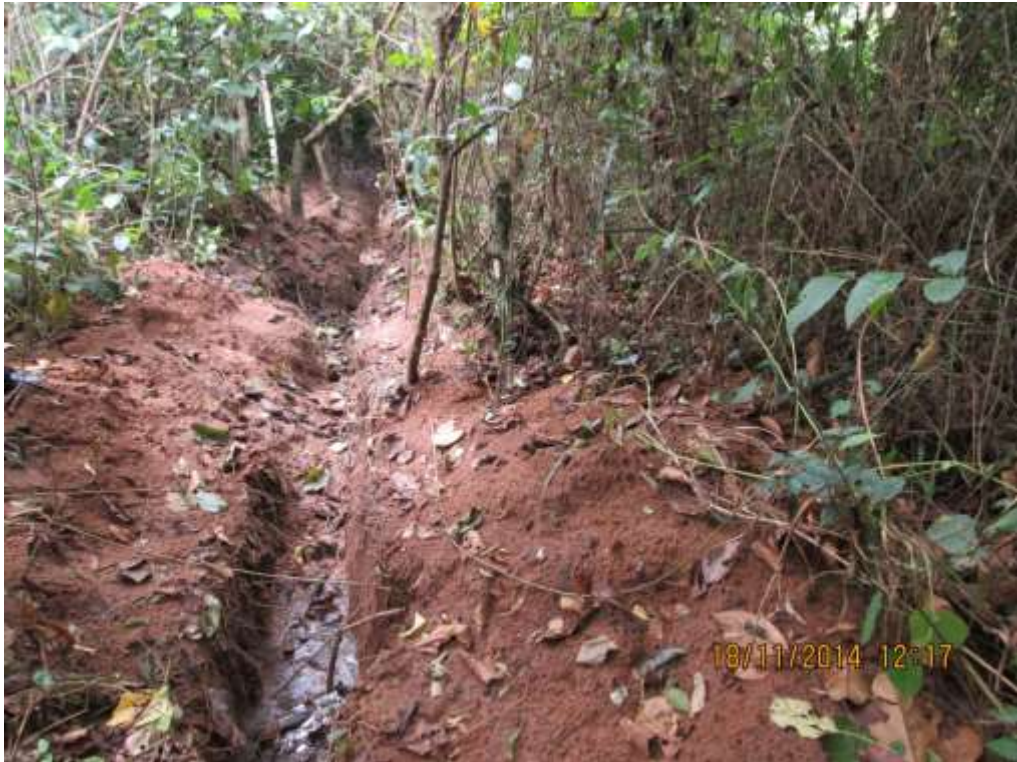
Overview: Site of spill on 4" Ahia Well3S Flowline Right of Way at Egbeda. Picture was taken during Joint Investigation of 18 th November 2014.
