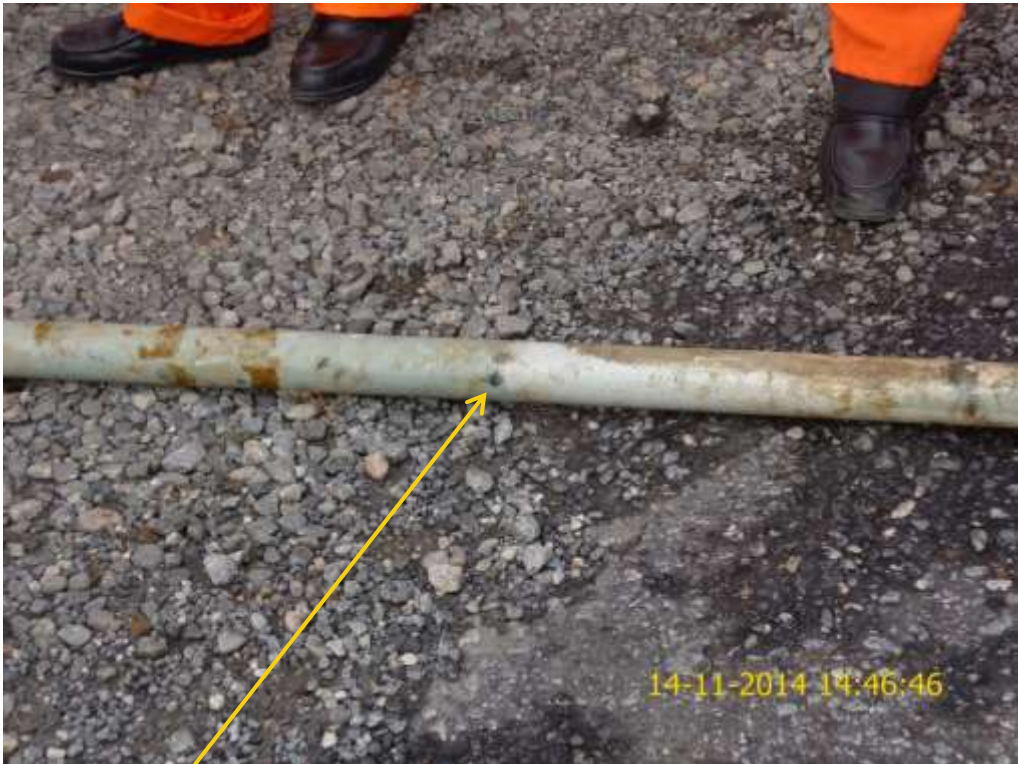
Close-up: Spill due to corrosion on Obigbo AGG Process Drain Vessel 2" Drainline at Umuebulu. Picture was taken during Joint Investigation of 14 th November 2014.
